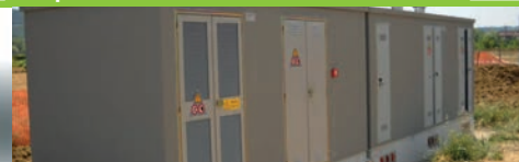
Telecontrollo cabine MT
