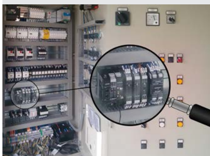
Control and command panel for underpasses with SENECA hardware and electromechanical redundancies
